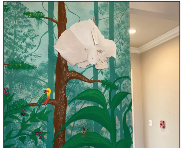
Damage to mural at Lackland Fisher House III
