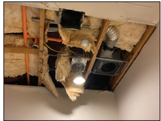
Water damage due to broken pipes
